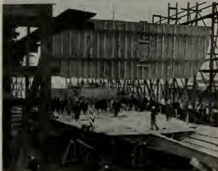
Keel-laying for the new steel auto passenger liner, at the Todd Shipyard Corporation Plant A, Seattle, Washington.
